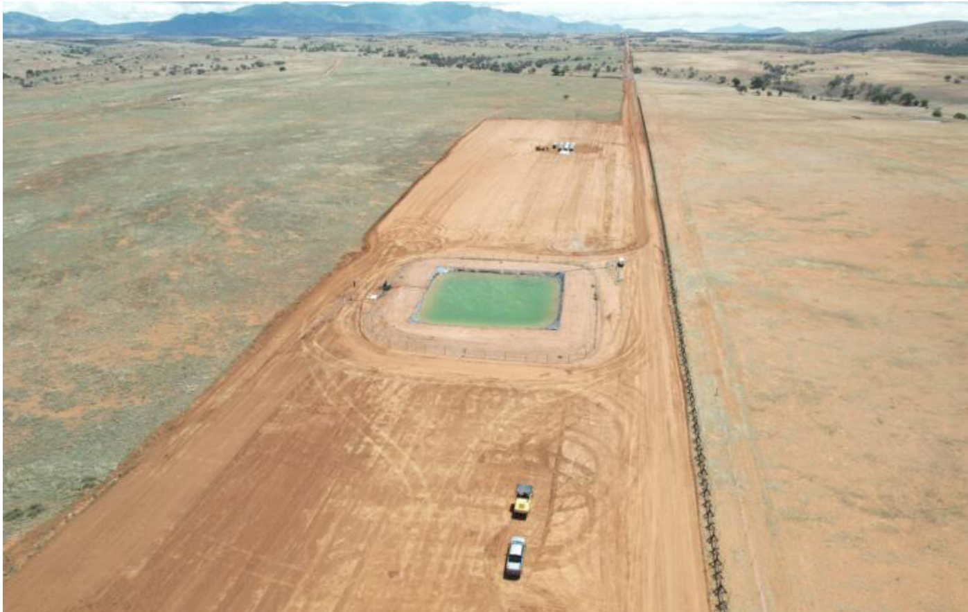
The site of a groundwater well in Arizona along the U.S.-Mexico border as seen from a drone. (Courtesy Myles Traphagen)
